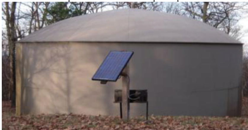
FIGURE 5.1 Small solar cell installation monitoring the water supply in Shenandoah National Park in Virginia.
